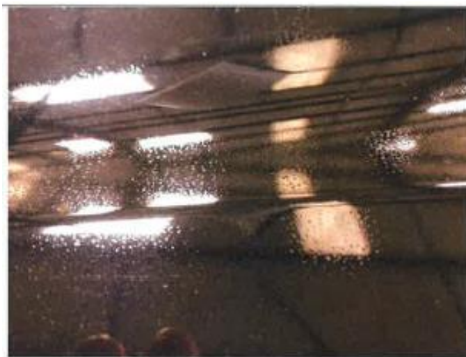
Close up of hood showing blistering
